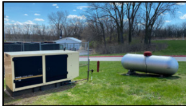
Ames High School (prior location)
